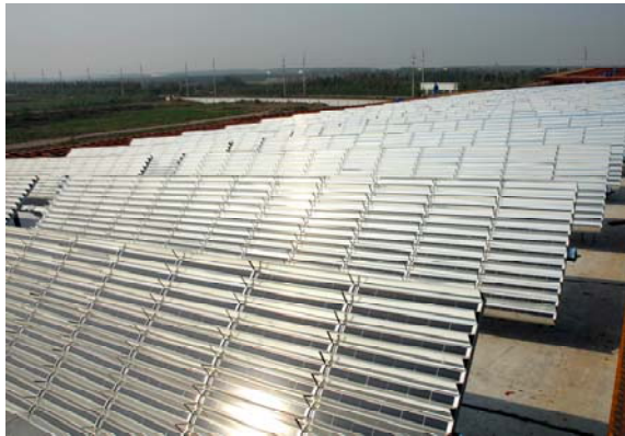
Figure 10: Photograph of 100 kW 3-sun array.
